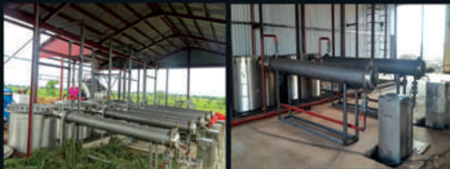
100 & 50 TPD Steam Distillation Plant
