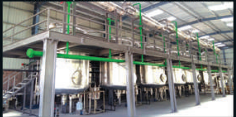
Turmeric (Curcumin) Extraction Plant
