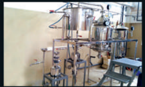
Pilot Scale Distillation Plant
