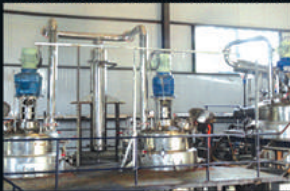
Natural Colours Extraction Plant
